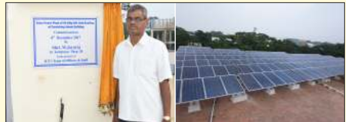
Solar power plant of 50 KWp ON-Grid rooftop was commissioned at Furnishing Admin Building on 08.12.2017 by Shri. M.Jayaraj , Sr.Tech/Shop-28, in the presence of ICF's Team of Officers and Staff.
